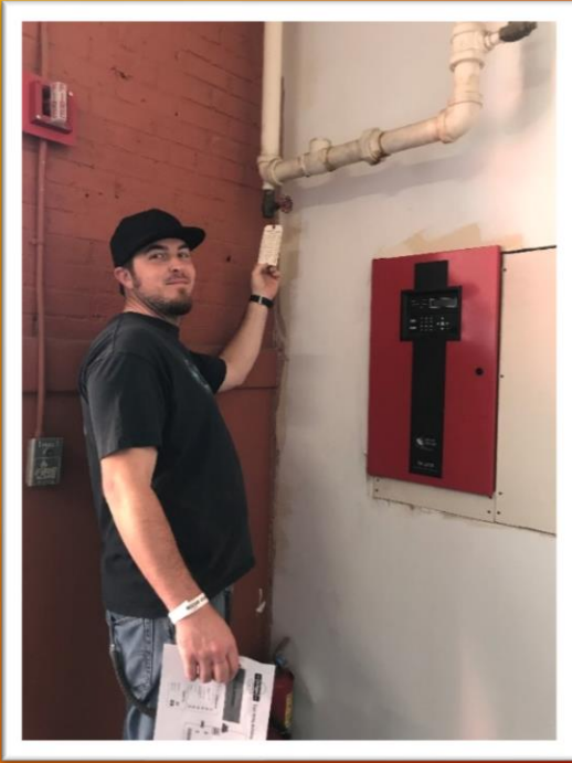
Paul, Sprinkler Service Foreman, checking service tags while visiting the Dr. Pepper Museum in Waco – always making fire and life safety a priority!
