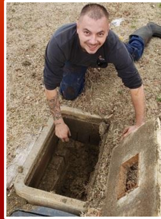
Stephen, Backflow Technician, working to repair and retest a failed backflow so our office can provide passing test results to the city for our valued customer.
